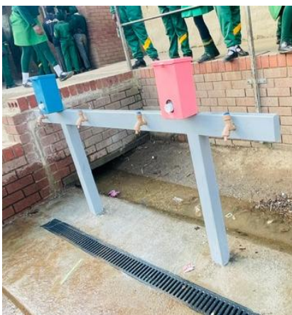
New drinking/hand washing fountain
